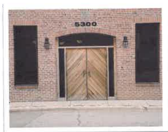
Figure 2.18: Discouraged Entryway – Opaque windows, and windows that do not make up the majority of the storefront give the appearance of a residential entryway rather than an entryway of a commercial building.
