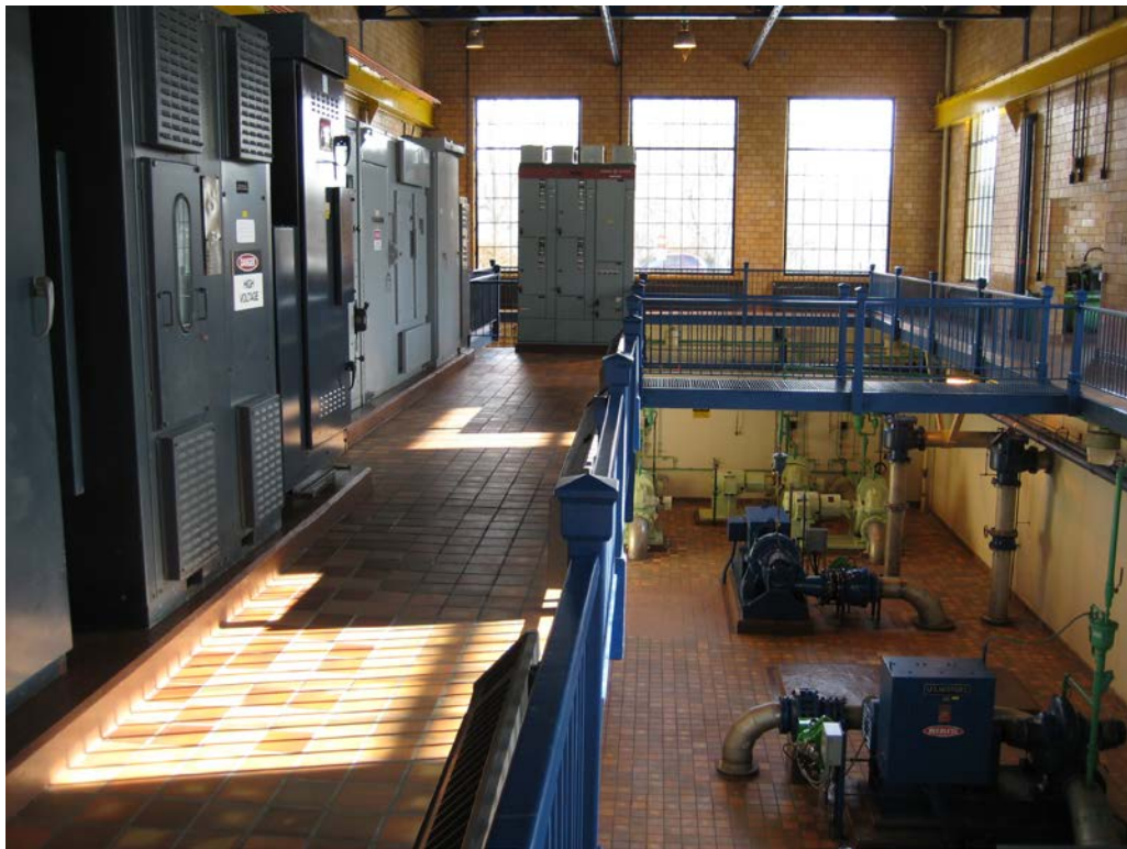
High service and low service pumping station
