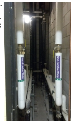
Purple pipes in Mechanical chase area of new Findlay City school.
