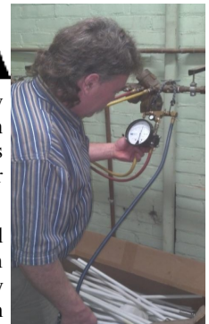
Eric Helms, Plumbing Inspector tests backflow devices at Traffic shop.
